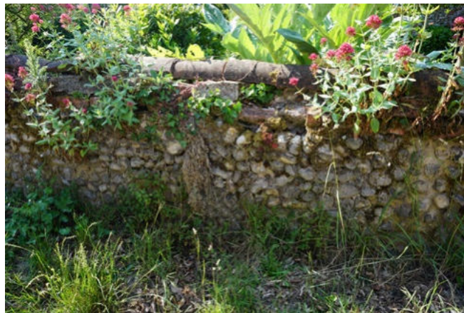
Vegetation growth to a wall, likely to be causing structural damage
