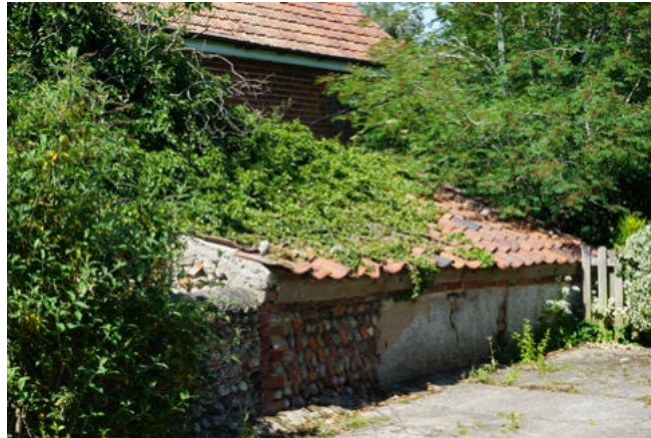
Outbuilding in poor condition with overgrown vegetation
